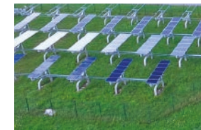
EDF Renouvelables Photovoltaic solar power station on trackers
